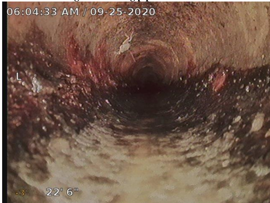
Photo 10 – Scaling and thinning pipe
