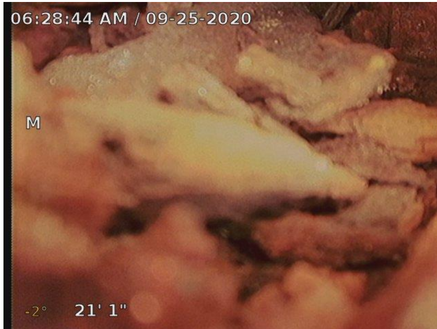
Photo 9 – Debris in the line
