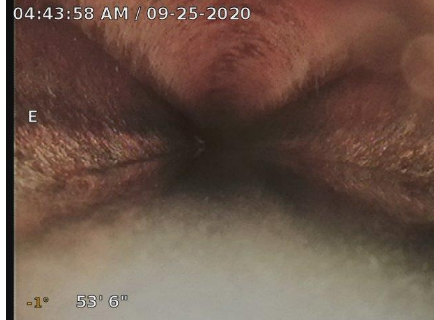
Photo 5 – Scaling pipe with standing wastewater
