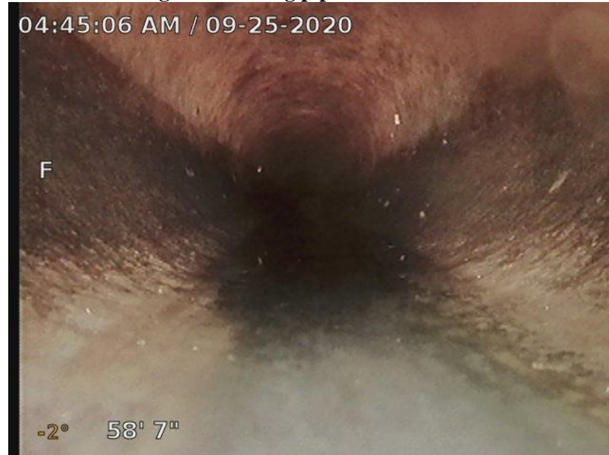
Photo 6 – Scaling and thinning pipe
