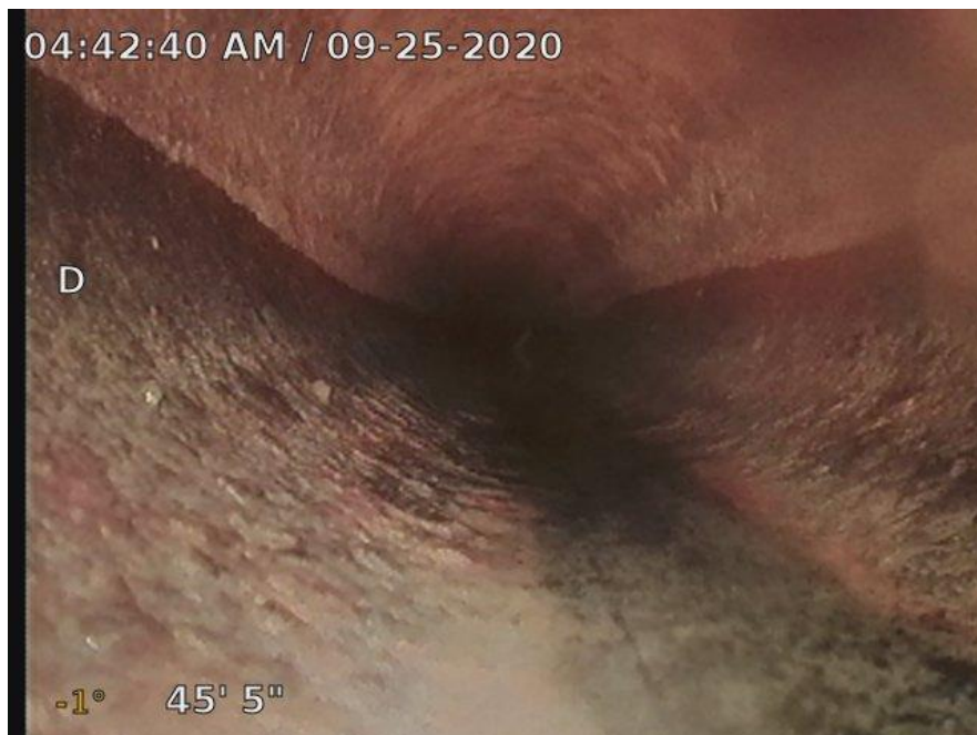
Photo 4 – Scaling and thinning pipe
